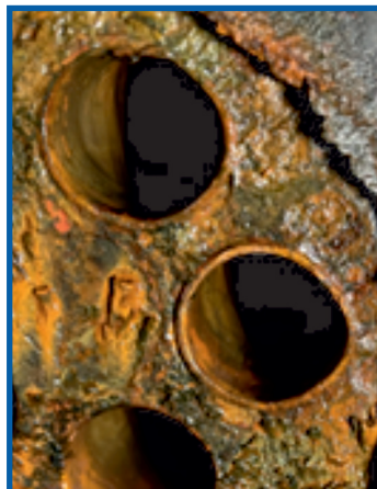
December 2020 - Scale build-up reduced
